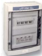
AC surge protector panel
